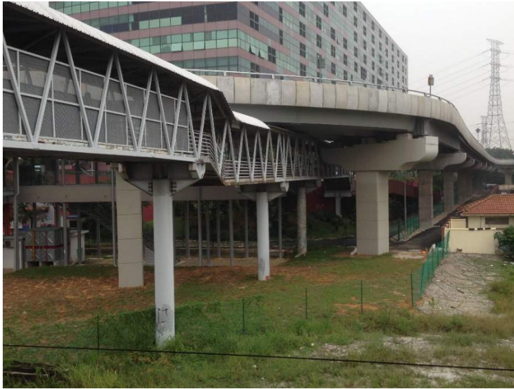
Figure 15 Showing the poor pedestrian access on the Mentari side. The link bridge is a better option.
